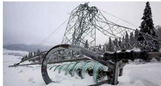
Fig. 3. Consequences of icing on a high-voltage overhead power line
