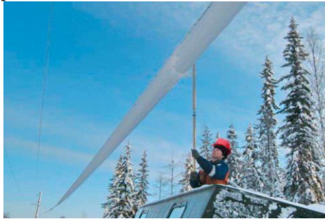
Fig. 8. Mechanical removal of ice from the wires of overhead power lines.
